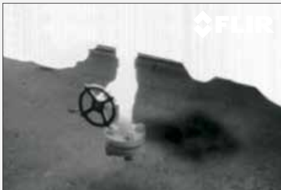
Methane leak at natural gas facility site.
